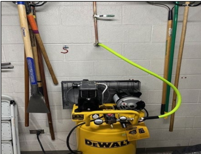
Station 151 compressor and plumbing
