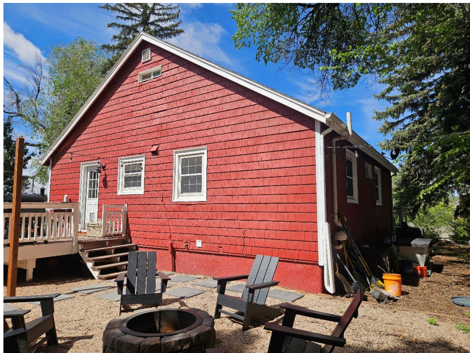
East and north elevations of the residence, view west (Roll 26-450, image 103249; Emily Wren; 5/22/2026)
