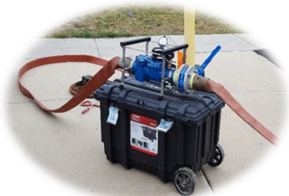
Mobile bench tester checking the flow on the 6-inch Justice Center meter
