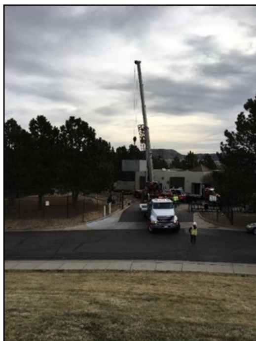
Meadows Water Treatment Plant
