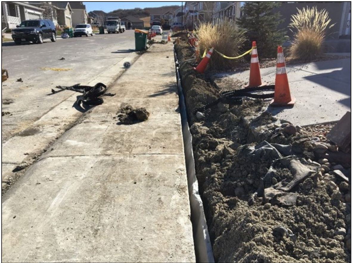
Underdrain in Trench behind Sidewalk on Starry Night Loop
