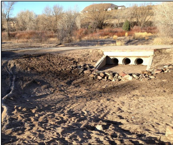
Before: 3-24" Culverts completely filled in with sediment following a June 2015 storm event
