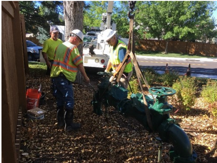
Old 6-inch backflow in place
