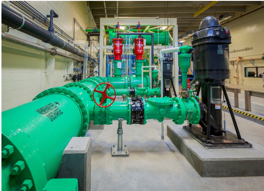
Modern Day Water Pipes
