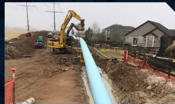
Drilling mud was used to keep the tunneled hole from collapsing and to lubricate the waterline as it was pulled into place.
