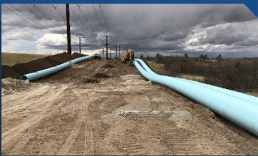
Rocky and steep terrain, combined with overhead powerlines, made pipeline installation difficult.
