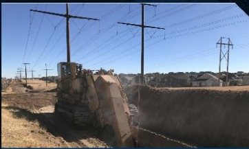
Specialized equipment was mobilized from Texas to cut the rock ahead of installation. This was a much safer method than blasting through the bedrock.
