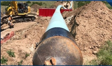
This metal drill head steered and guided trenchless installation of the waterline.
