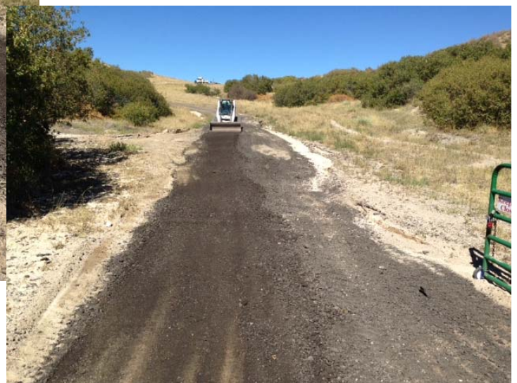
Asphalt millings were added to increase the durability of this dirt road.
