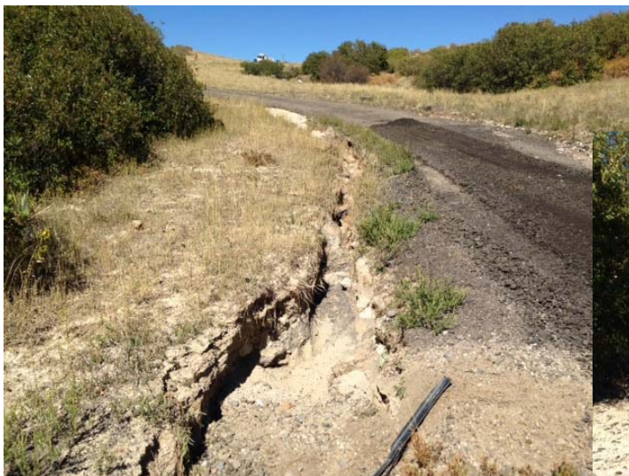
Water erosion on Reservoir 17 Road.
