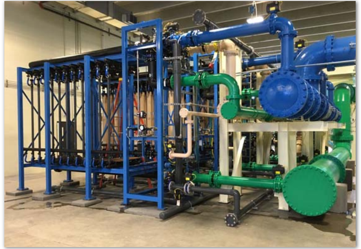
The membrane expansion is the heart of our new Plum Creek Water Purification Facility.
