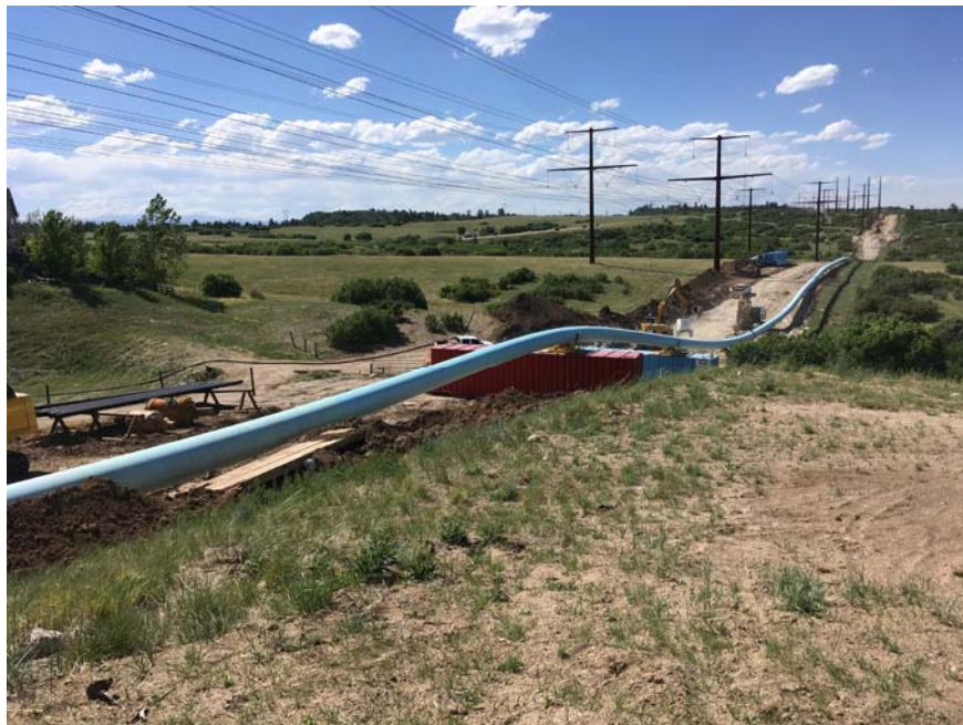
The WISE pipeline - a critical piece to ensuring a sustainable water supply.
