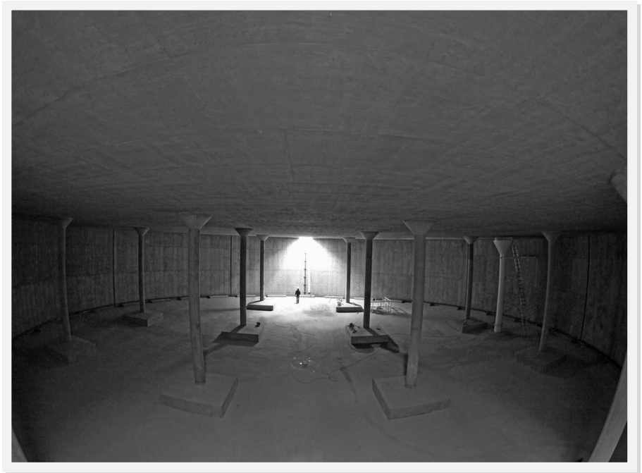
Inside of a water tank after completing construction. In Castle Rock, the total storage volume available is 35.6 million gallons which balances daily demands with potential emergency needs.
