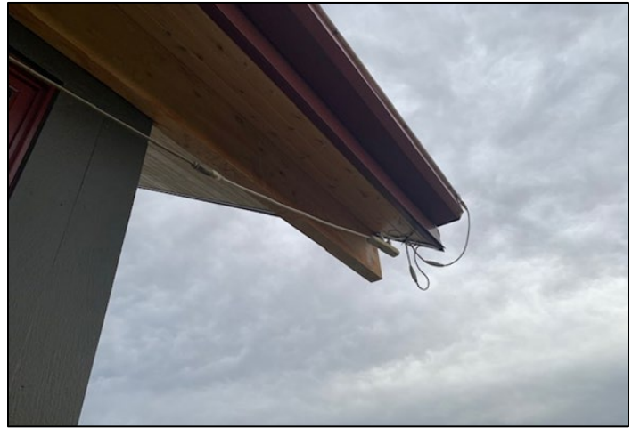
Inspection; an indoor surge protector used for outdoor lighting
