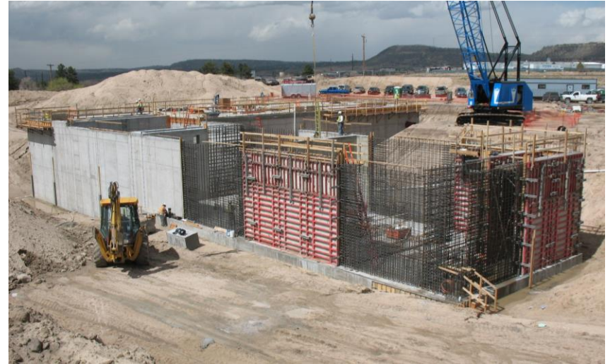
Construction of Existing Pretreatment Basins in 2012 New Pretreatment train to add 6 MGD capacity
