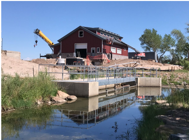
Sedalia Pump Station
