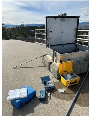
Testing kit at one of the storage tanks.
