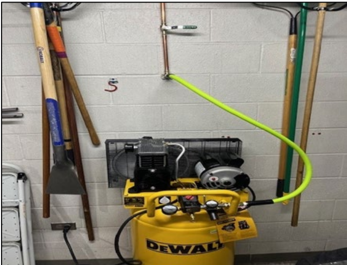
Station 151 compressor and plumbing
