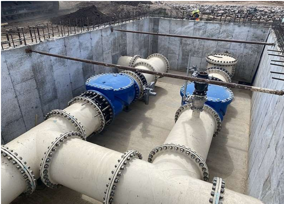
Castle rock Reservoir #2: Vault and new piping
