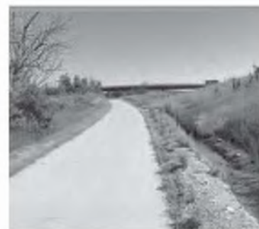
An eroded and ponded channel adjacent to the trail leading from an outfall from I-25. If practical, a remedy to this drainage issue to get the flows under the trail will be incorporated into the design.
