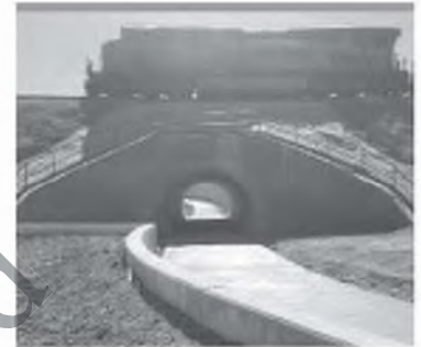
The Fossil Creek Pedestrian Tunnel (Lithos staff experience) spans 70 linear feet underneath BNSF.
