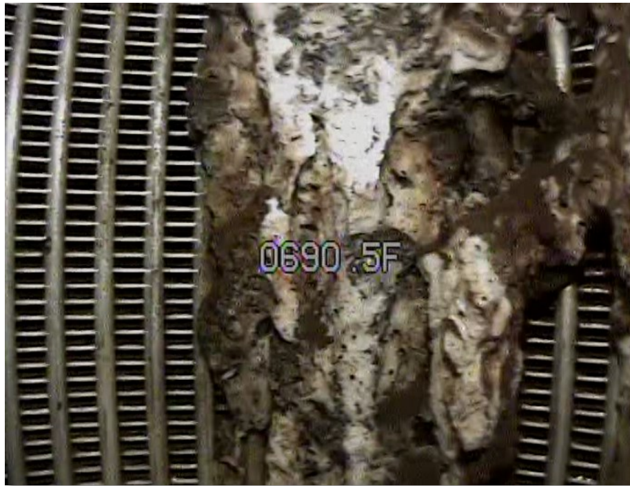
Well video image showing the calcium bridge at 690.5 feet below the surface after the first round of rehabilitation
