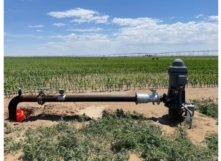
Typical Lost Creek Basin well structure
