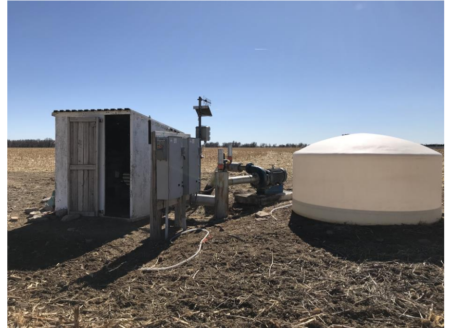
Typical Lost Creek Basin well structure
