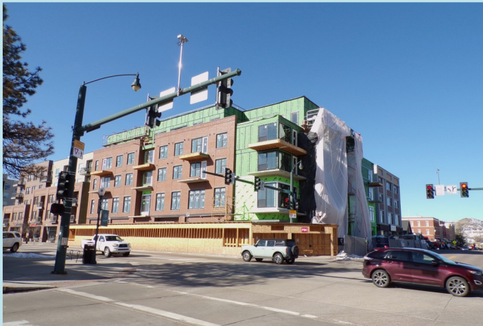
221 N. Wilcox Street, Riverwalk Luxe Landscape design revision to include bike racks along Wilcox Street in paver zone.
