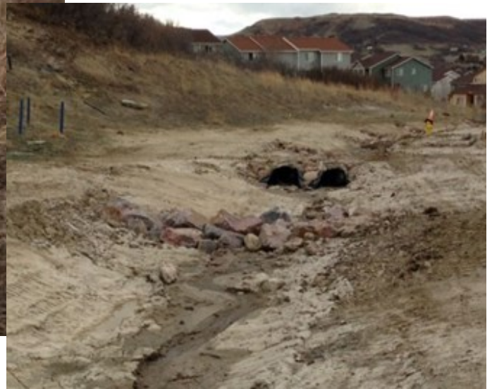
Repairs made to the Plum Creek Ditch after it had become clogged with sediment, plants and debris, causing it to spill onto Plum Creek Parkway during severe storms. This overflow created road icing, which was a safety hazard for drivers on this main arterial.
