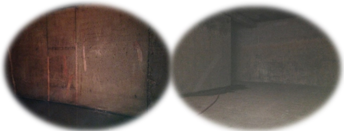
The clear well at Plum Creek Water Purification Facility was cleaned and sanitized.
