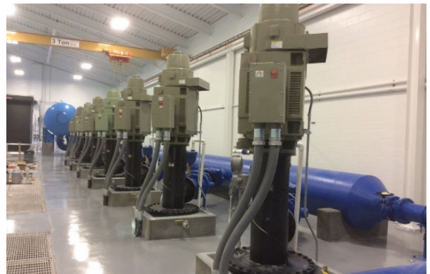
Canned vertical pumps at the Donkey Creek Pump Station in Gillette, WY.
