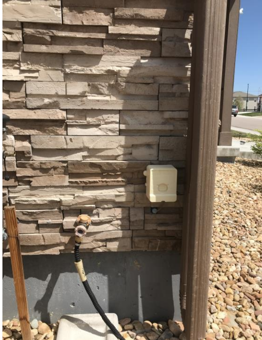
Radios are on Side of House
