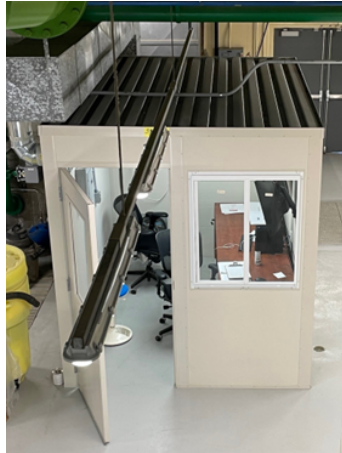
New Control Room
