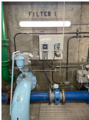
New actuators and transmitters
