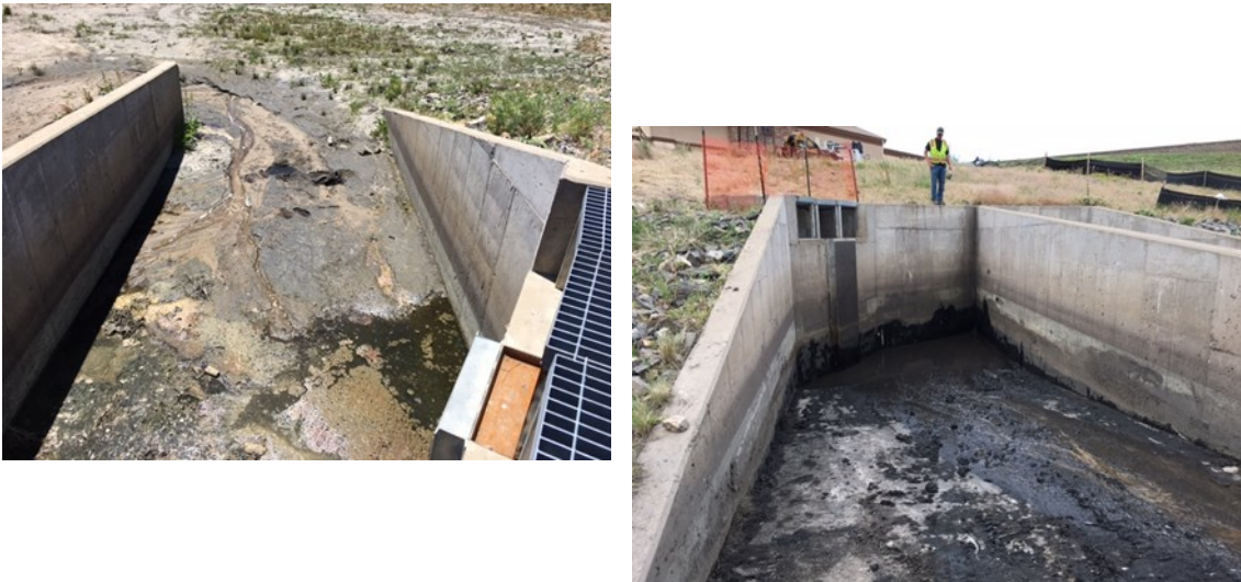
The Stormwater Team used the Vac Truck to remove algae, sediment and debris from the Lowe’s stormwater pond outfall. Their work will enable proper flow and reduce mosquito breeding conditions.
