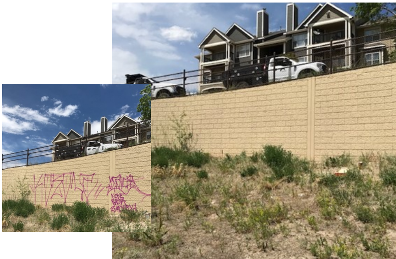
Unwanted art removed in the Meadows by the Stormwater Team
