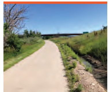
An eroded and ponded channel adjacent to the trail leading from an outfall from I-25. If practical, a remedy to this drainage issue to get the flows under the trail will be incorporated into the design.
