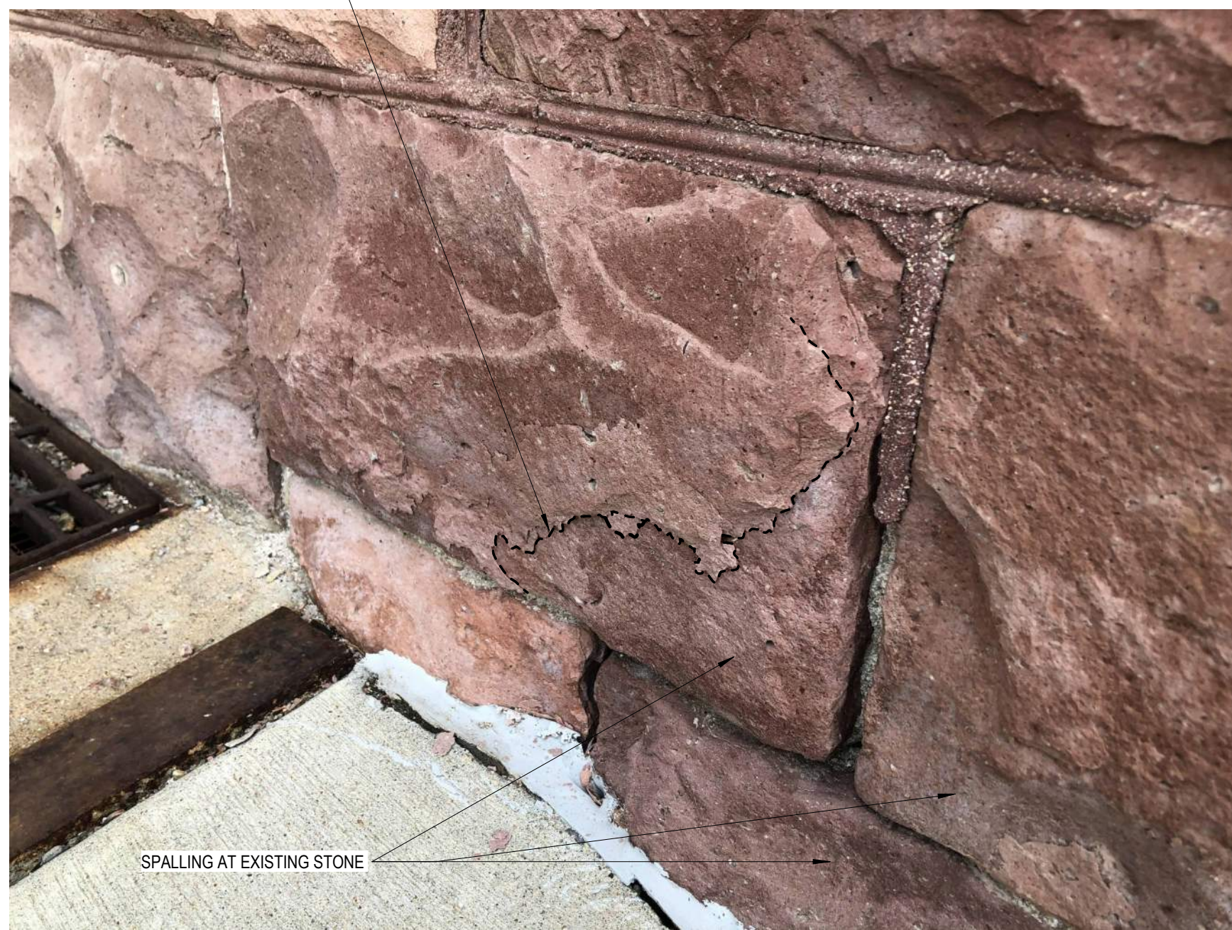
D6 STONE SPALLING & FLAKING NTS
