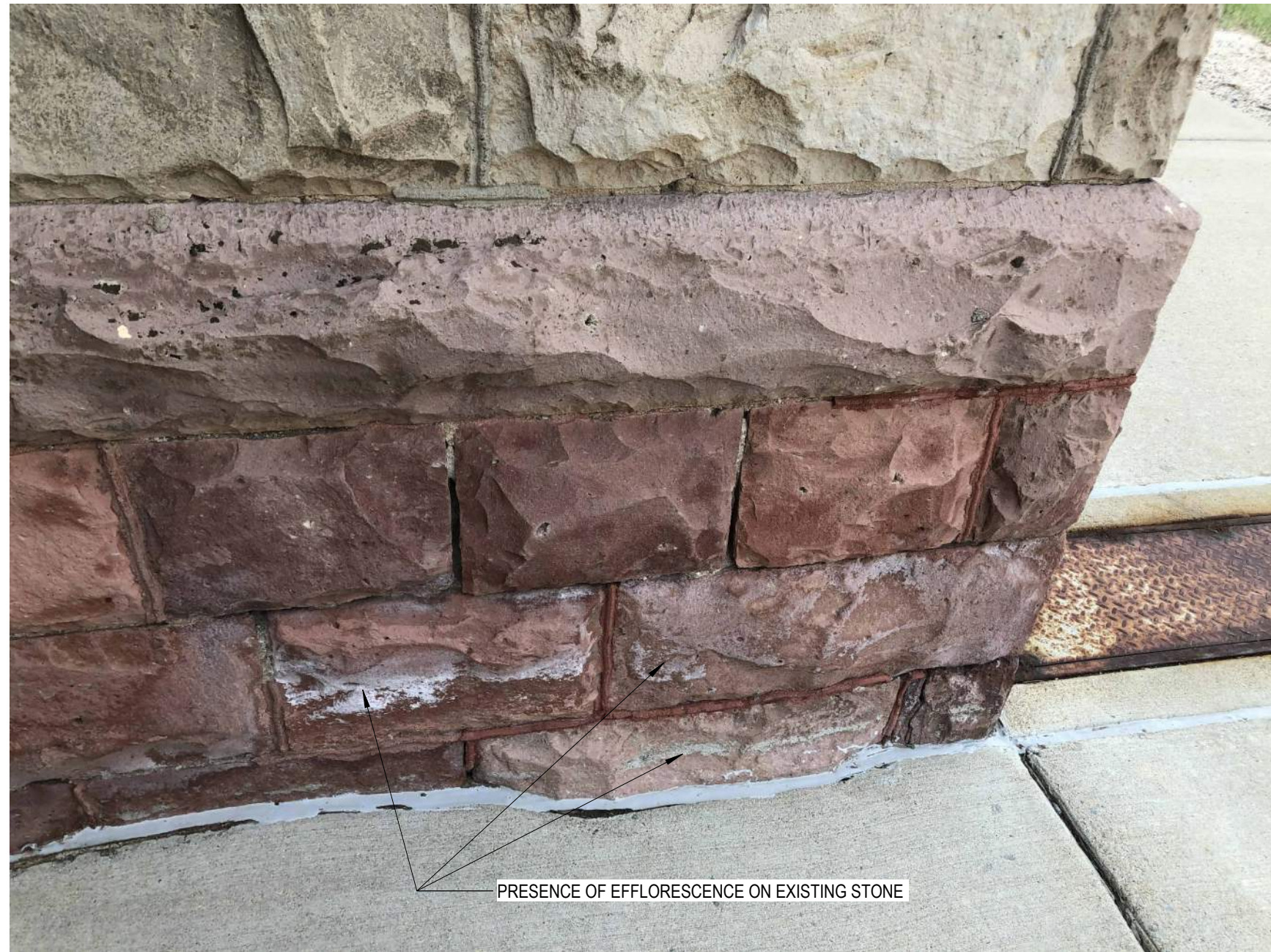
B3 EFFLORESCENCE NTS
