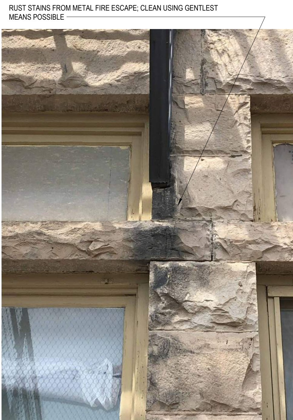
B1 STONE STAINING AT FIRE ESCAPE NTS
