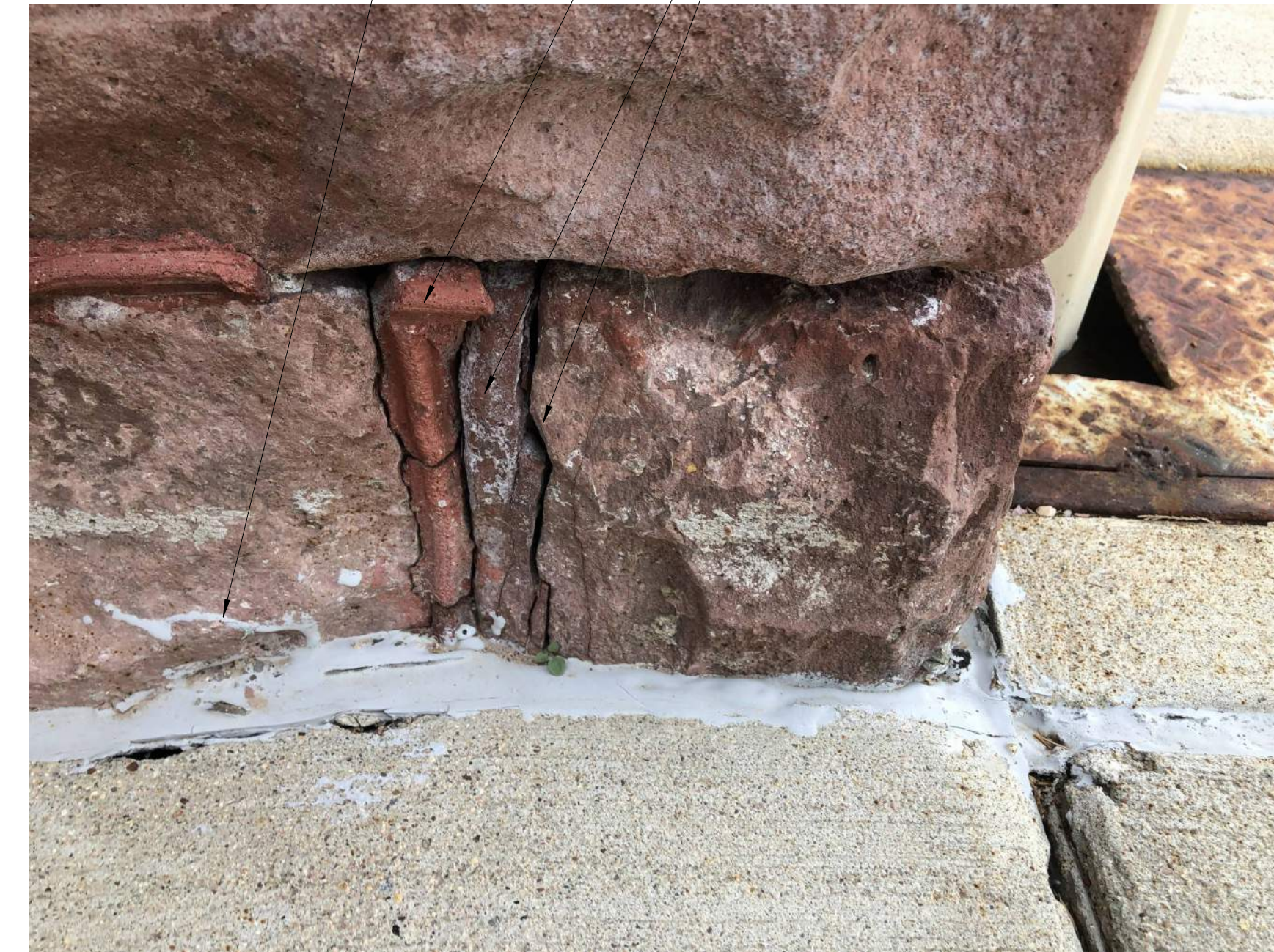
B1 CRACK & MISSING MORTAR JOINTS NTS
