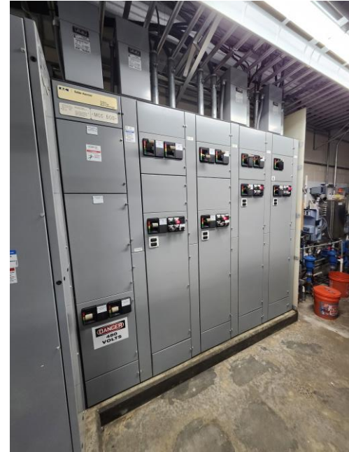
Motor Control Center
