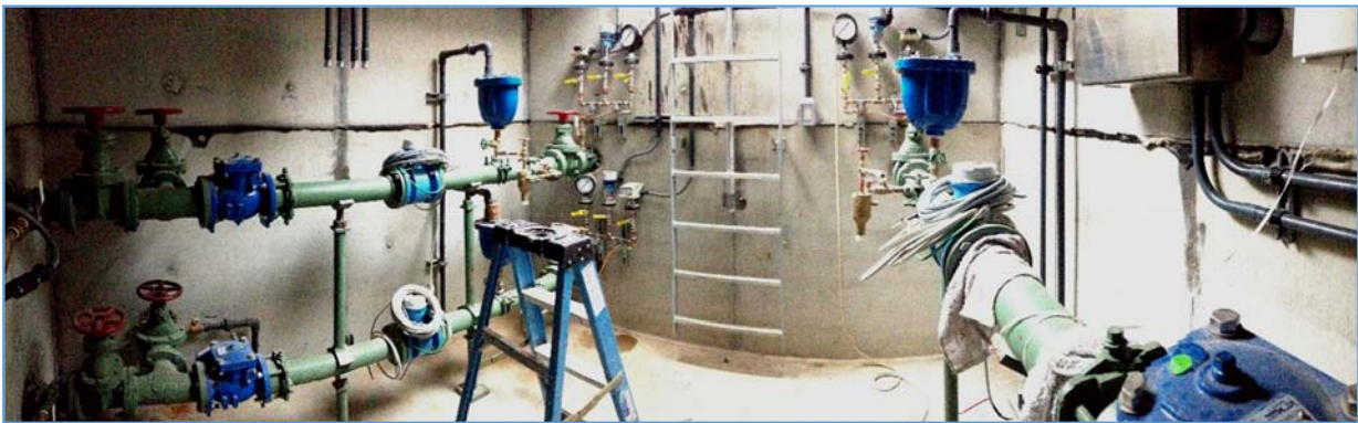
AL-16, AL-18, and AL-20 metering vault.
