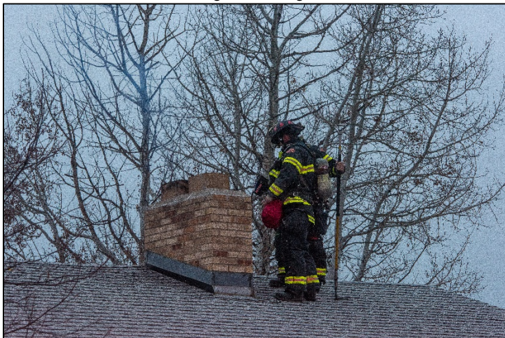
Assessing the damage
