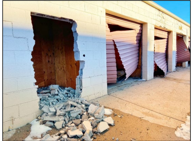
Breaching at Jerry Street acquired structure
