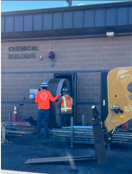
FRP tank rings being rolled through the door of the chemical room...
