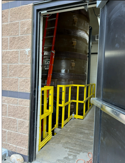
...and the fabricated tank in place. It is so large it's difficult to get a good picture of the tank inside the room!
