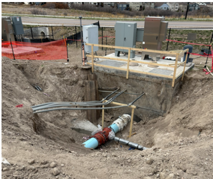
The tie-in of the new 6-inch red zone line into the 18-inch WISE line that routes into the clearwell.
