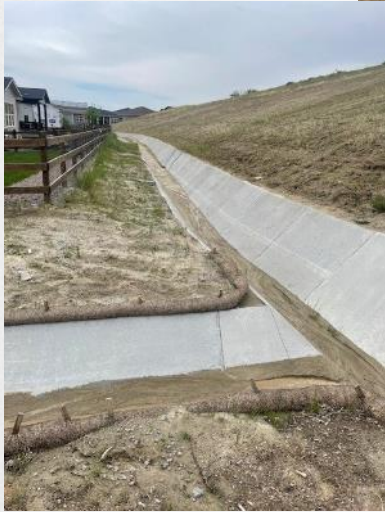
Drainage channels protecting homes in Lanterns
