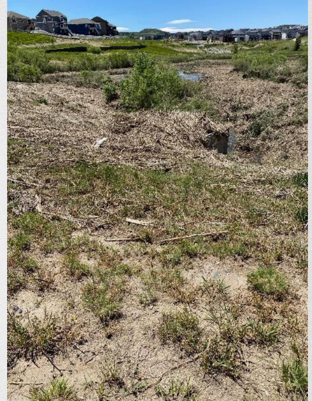
Regional detention pond in Crystal Valley with debris lines at approximately 100-year volume
